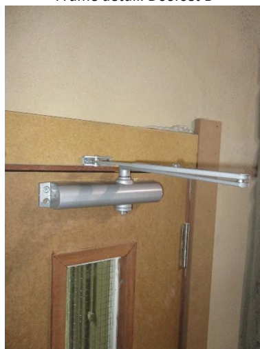
-Door closer detail. Doorset B-
